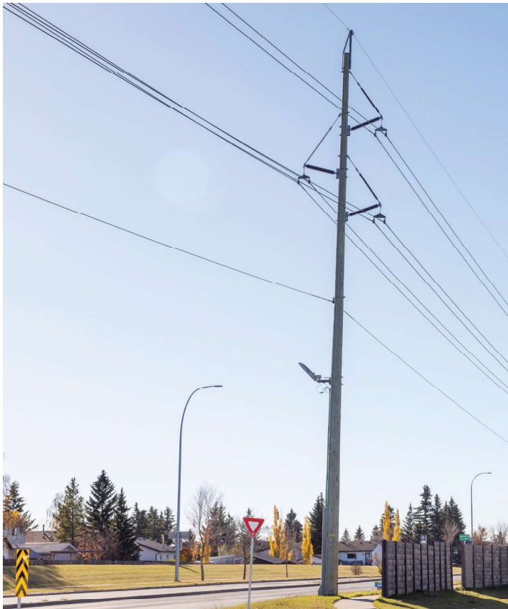
Example of Existing Wood Pole
