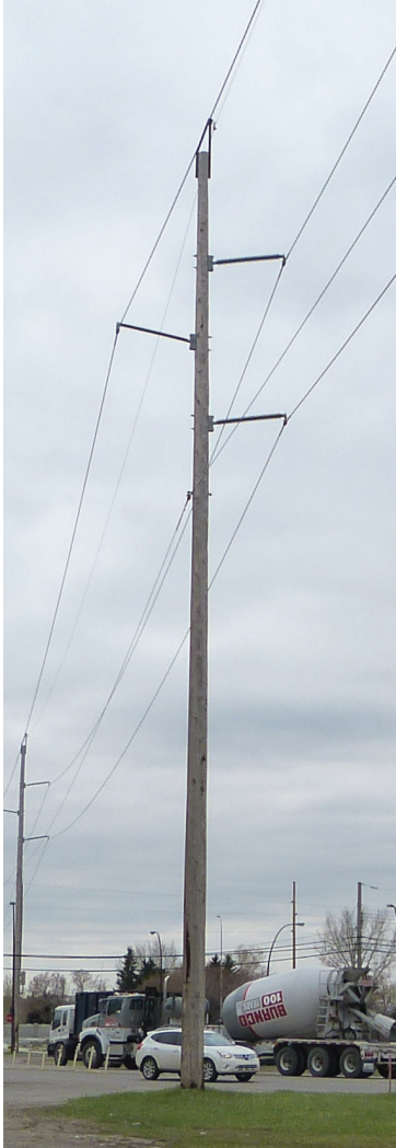
Example of Wood Pole
