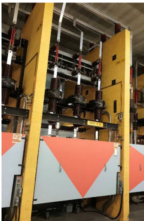
Example of Current Switchgear
