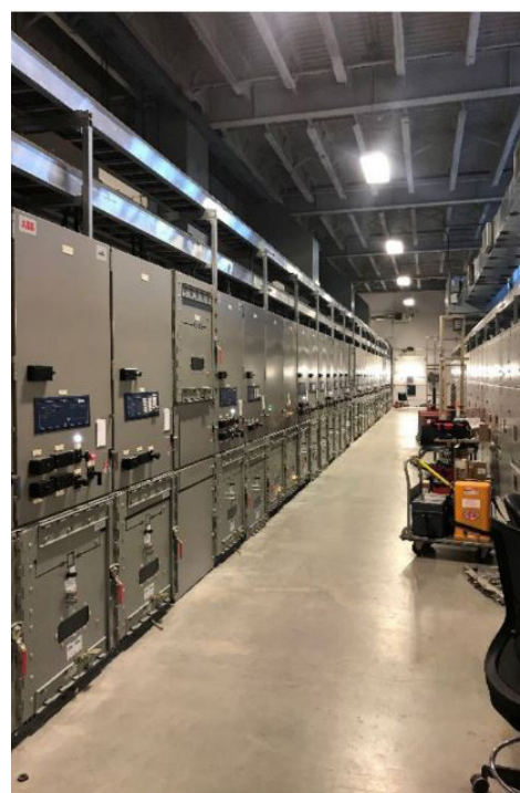
Example of Proposed Switchgear
