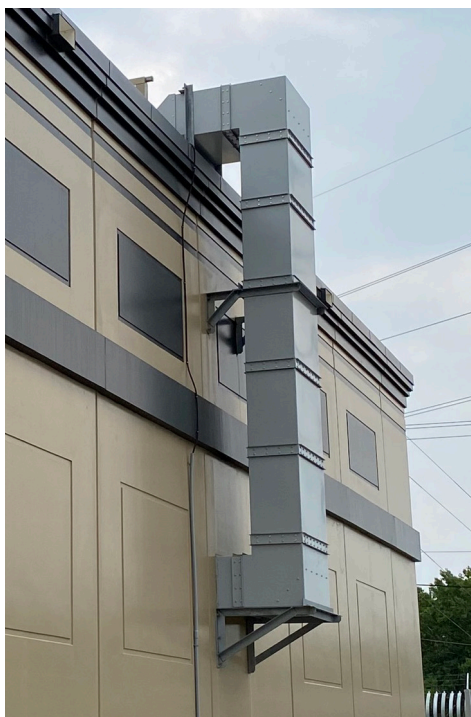
Example of Plenum Vent
