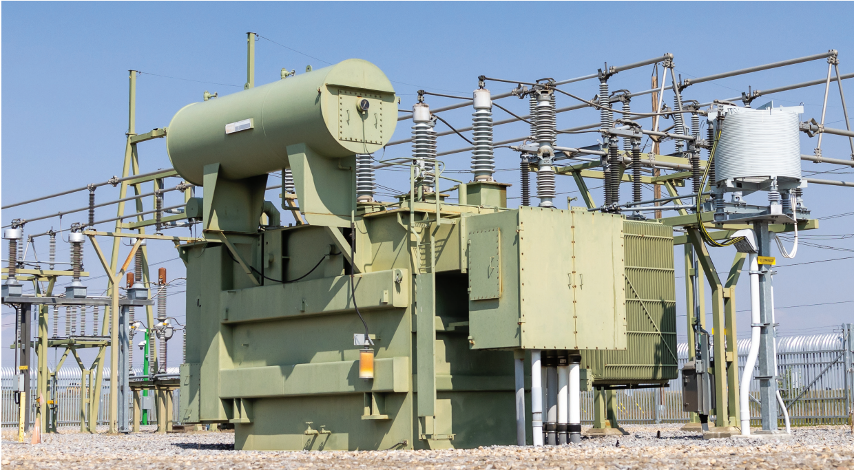
Example of Transformer
