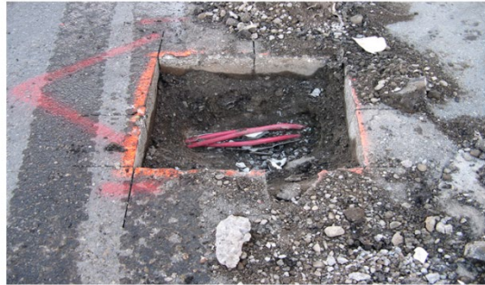
Shallow Cables in Downtown Network
