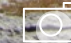
ENMAX Power field services crew installing poles and power lines at the Tsuut'ina Nation. Safety equipment includes rubber gloves and sleeves, hard hats, safety glasses, steel-toed boots, fire-retardant and high-visibility clothing and fall protection harnesses.
