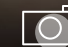
An ENMAX Energy team member checking water instrumentation at Shepard Energy Centre. Safety equipment includes hearing protection, safety glasses, fire-retardant clothing, hard hat and steel-toed boots.
