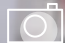
An ENMAX Power network civil crew completing maintenance on a network vault. Safety equipment includes fire-retardant clothing, safety flash protection glasses, safety gloves and steel-toed boots. The worksite is enclosed and high-visibility clothing is not required.
