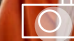
ENMAX Power civil crew connecting ductwork to a new underground vault. Safety equipment includes hard hats, safety glasses, cut-resistant class 4 gloves and steel-toed boots. High-visibility clothing is not required in this area as the worksite is enclosed.
