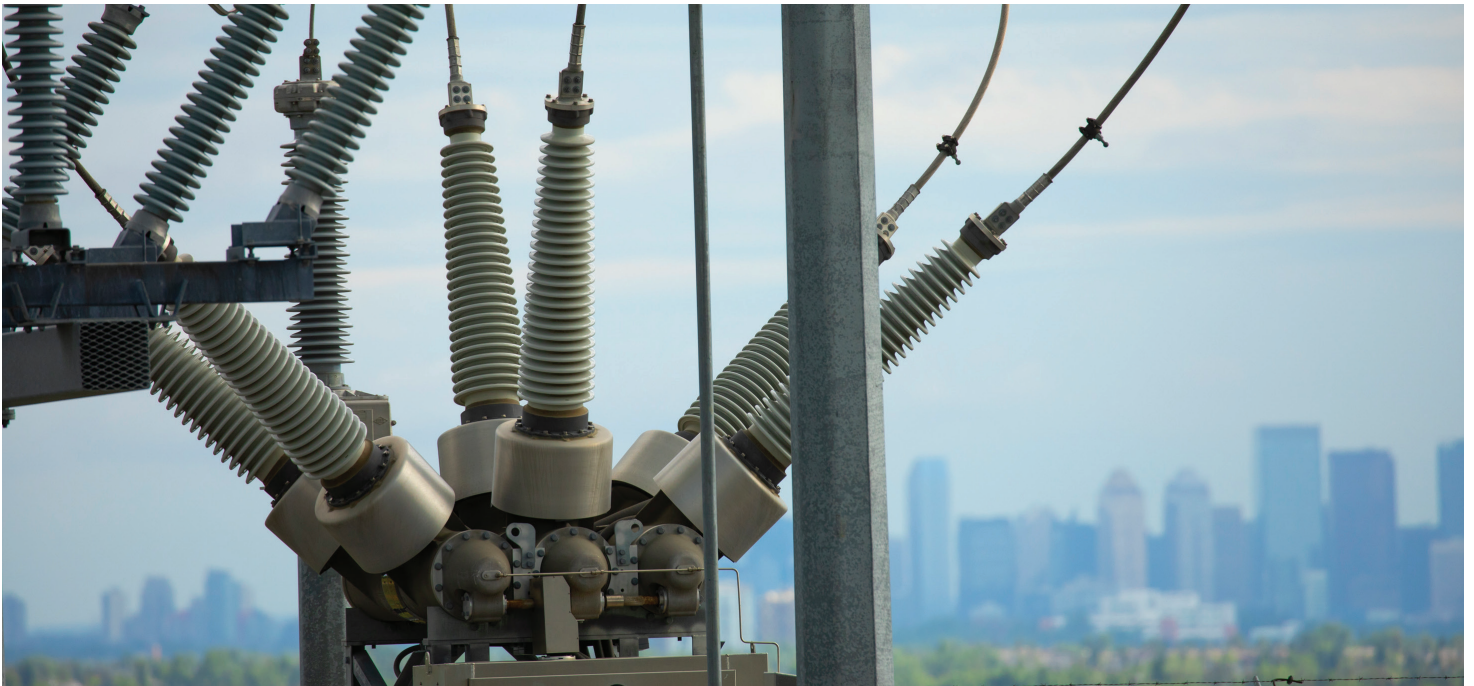
Example of a Circuit Breaker
