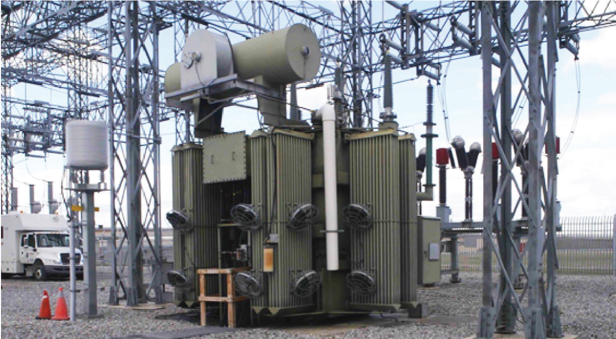
Example of Transformer
