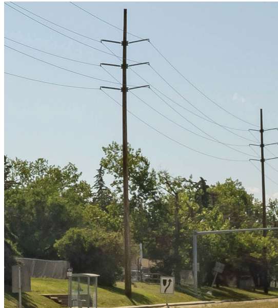
Example of Wood Pole
